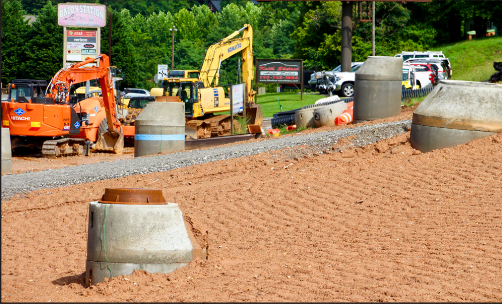
Slowly but surely, the area that opened up in a sinkhole last August is starting to resemble its former state at the intersection of Murphy Hwy and GA 515. Photo by Shawn Jarrard
